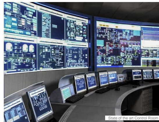
State of the art Control Room
